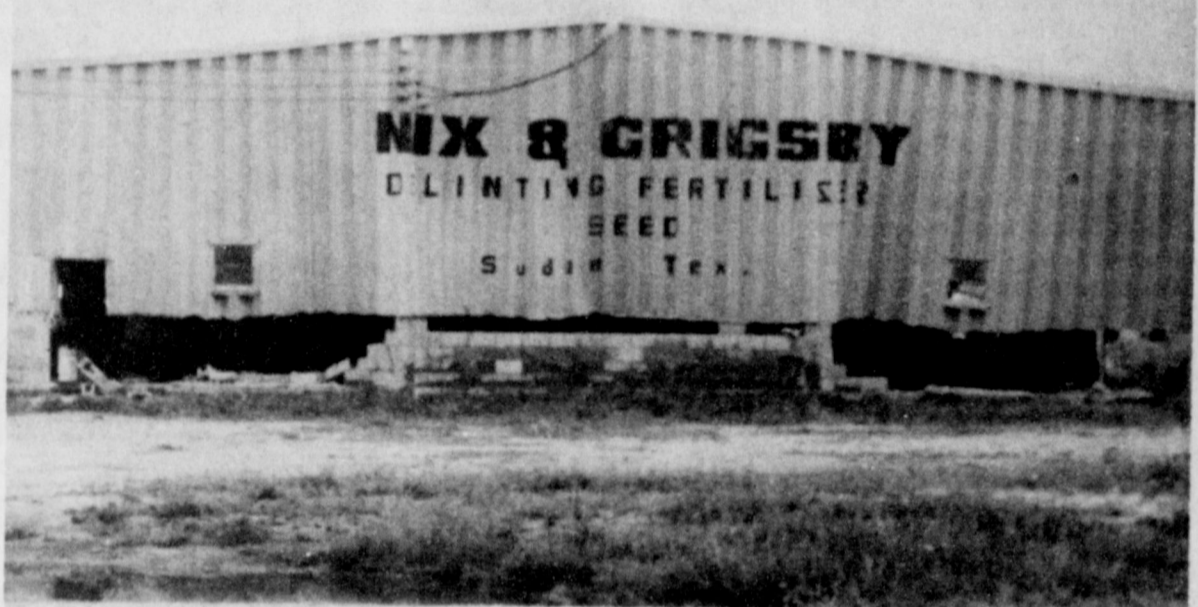
MINUS FOUNDATION--Nix and Grigsby firm at Sudan is minus the brick foundation to the front of their building. The twister, in its mysterious way of upsetting things, left the building standing, but took away the foundation.
