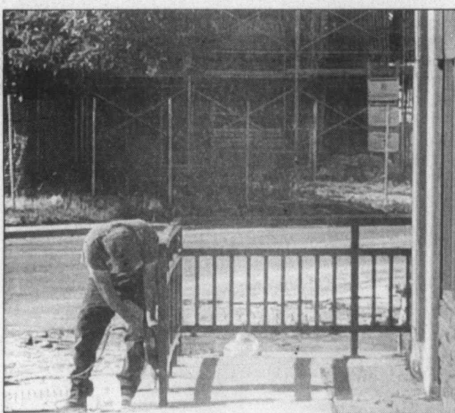
New railing ... Workers install a new railing around the sidewalk on the south corner of the 1600 block of Main Street, where a new handicap access area has been added.
