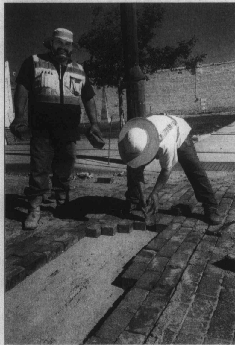
Re-laying history brick-by-brick ... Ryan Rodriguez (left) and Ricky McBride, with Cemtech Concrete company, were laying brick in the street just north of the Lynn County News office last week, replacing the historical bricks after they had been dug up for laying Tahoka water lines in the city waterline replacement project. After the bricks were removed for laying the pipelines, workers spent several days cleaning the old mortar or concrete off the sides of each and every brick, before it was relaid in the street. Upon closer inspection of the bricks, the News staff discovered the words "Thurber Brick Co." engraved on them, which, as it turns out, is a whole other piece of history about a town that now exists only as a "ghost town." (LCN PHOTO by Juanell Jones)
