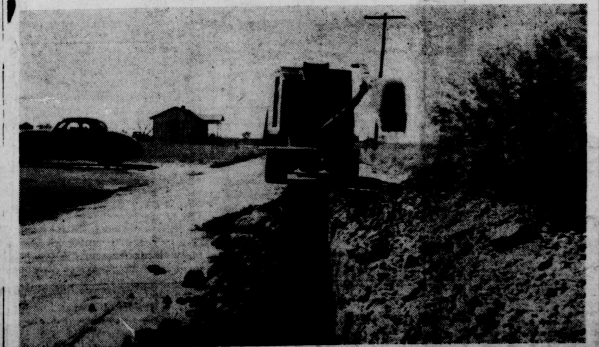
Shown in this picture is one of the City's maintenance units, a Quick-Way Fill and Ditching Machine. This unit has more than repaid its original cost in the current water and sewer extension project. Department employees who operate the machine are Leon Ivy and Chas. Adkins.
