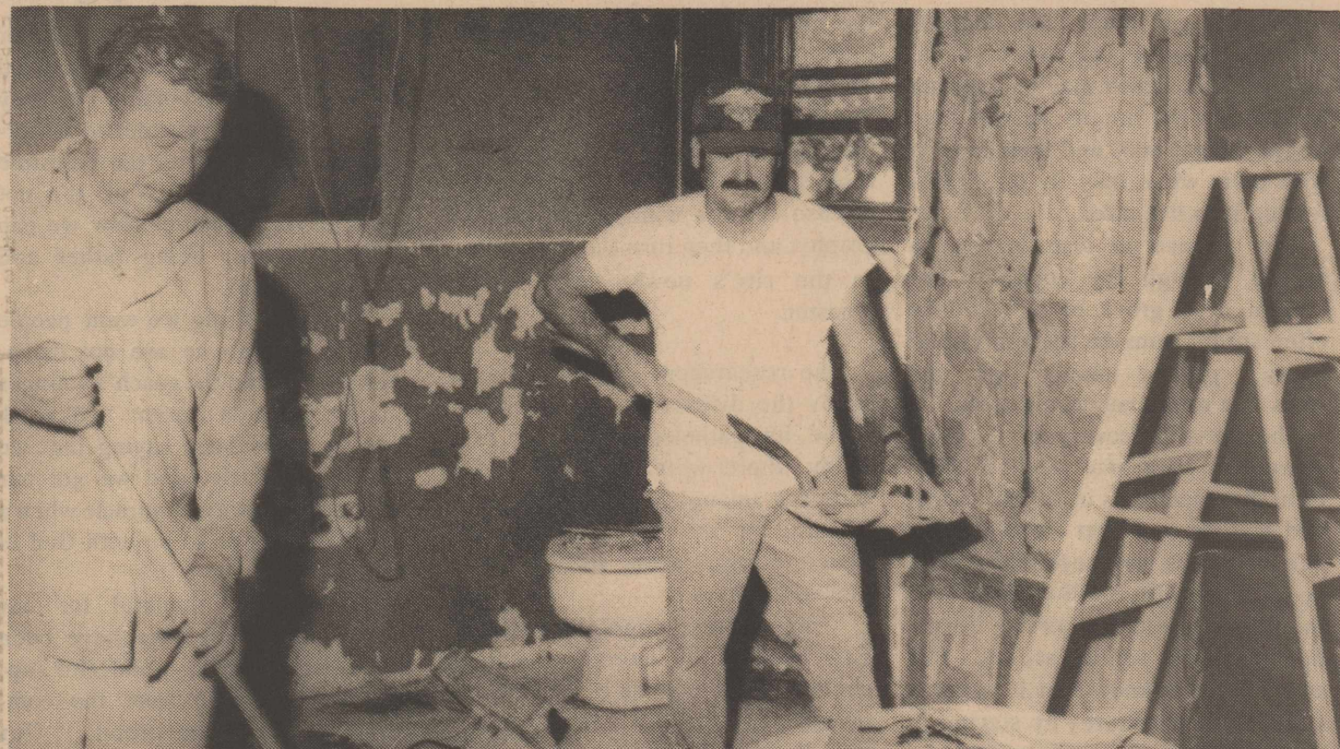
Homeowner Joe Lara [r] and his brother-in-law, Joe Rebelez, along with other family members and friends are clearing out the debris from the Lara's home. The structure was heavily damaged by a fire which began in the laundry area.
