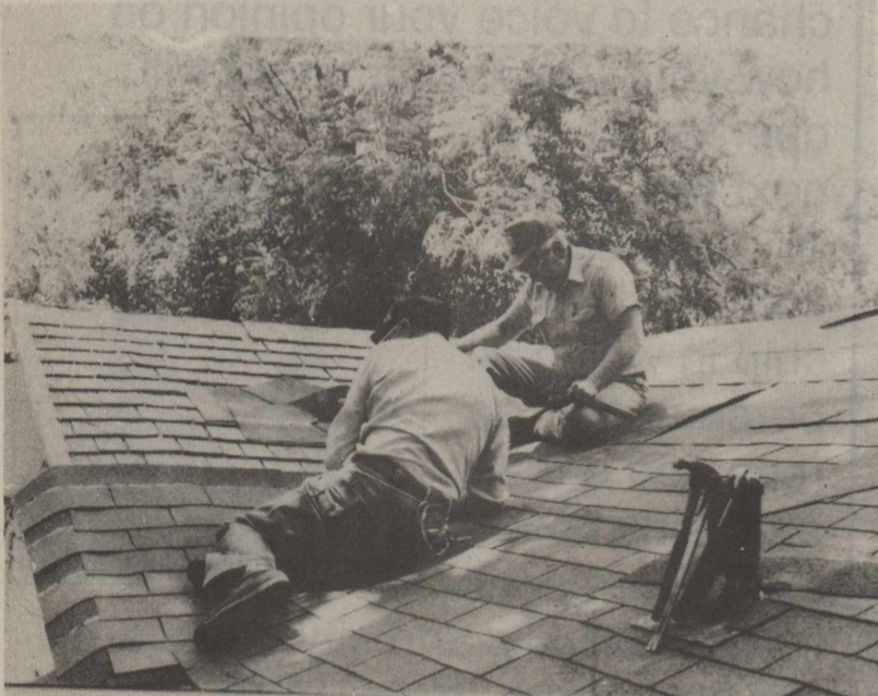
Bob Mooney and Stanley Mayfield work hard to finish shingling this roof Saturday.
