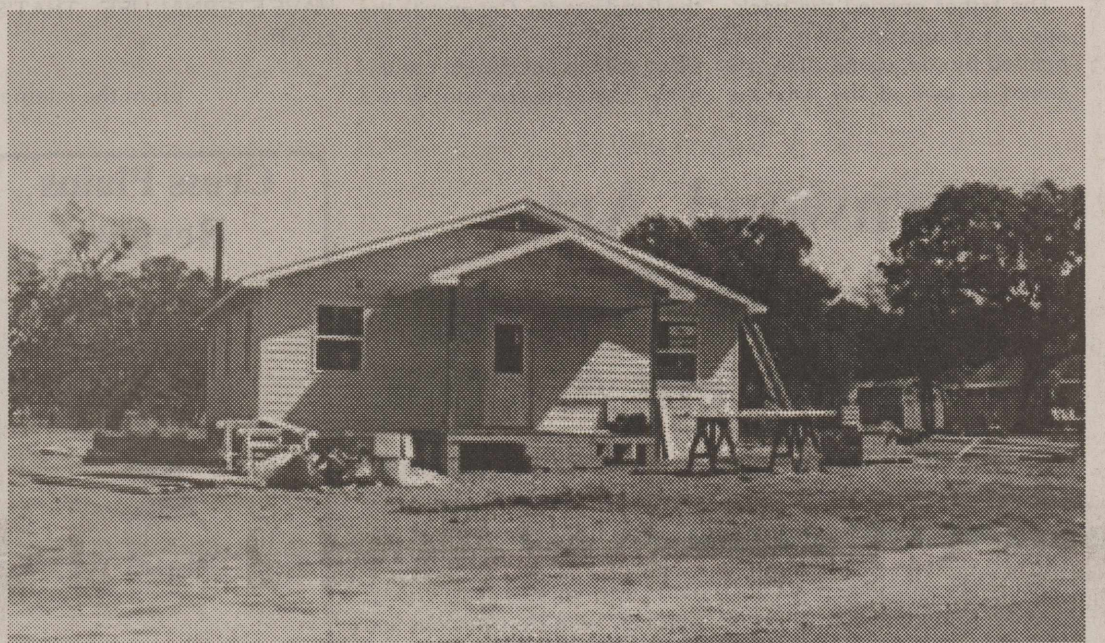
CAROL SAVELL'S NEW HOUSE May Baptist Church provided the materials and labor of love.
