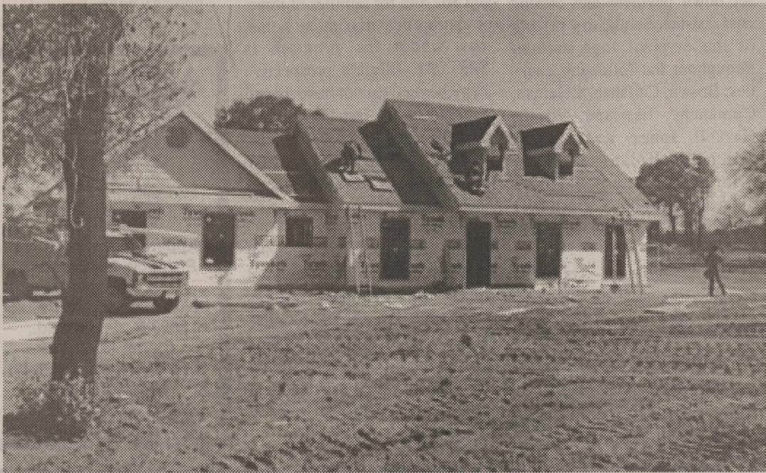
DAVID AND JANE HOLMES NEW HOME Cowboy Homes of Abilene are constructing this house.
