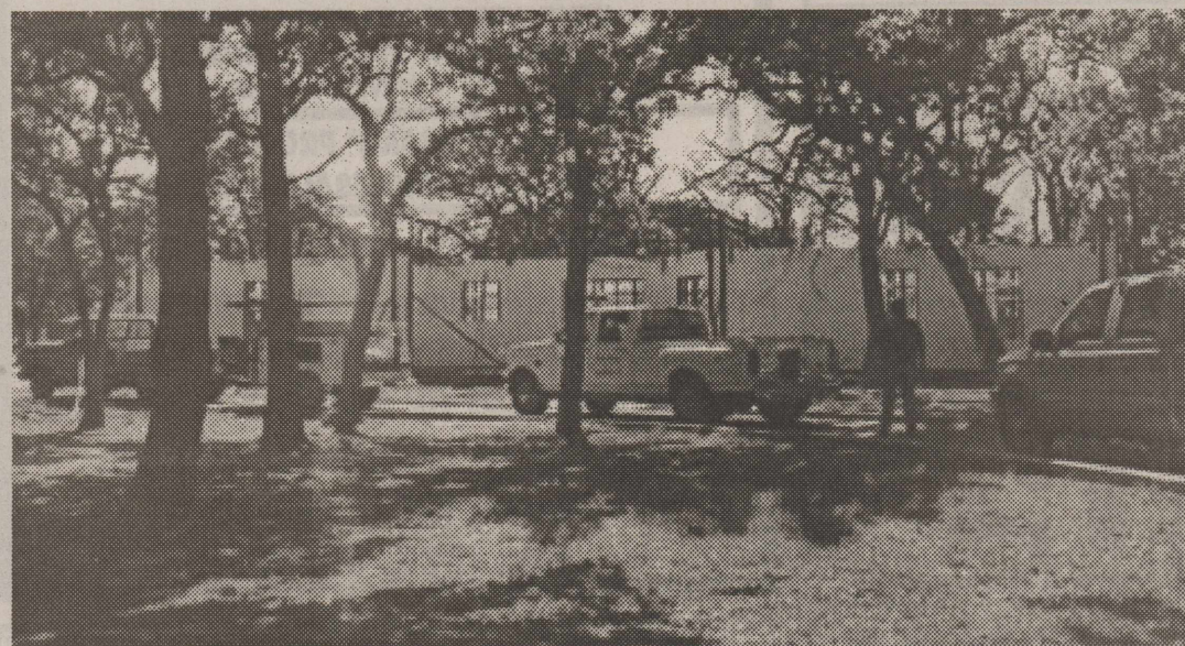
BUILT FOR GREAT INSULATION Styrofoam blocks were filled with concrete at the Chesshir house.
