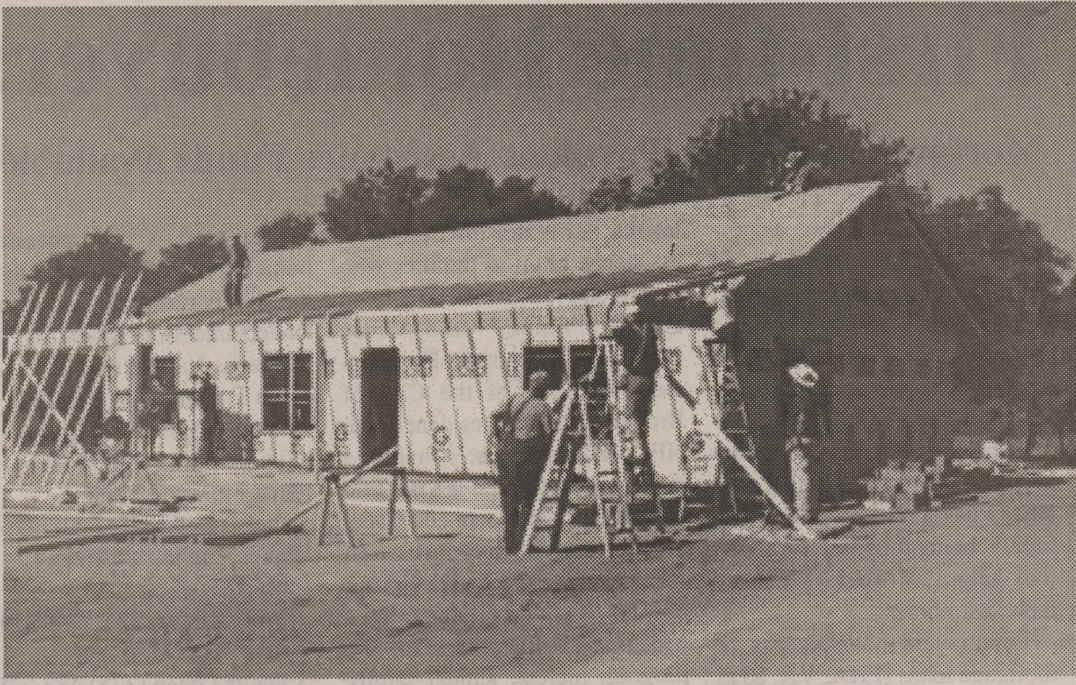
BAPTIST MEN'S MISSION AT WORK Retired builders are working on Nora Odom's house.
