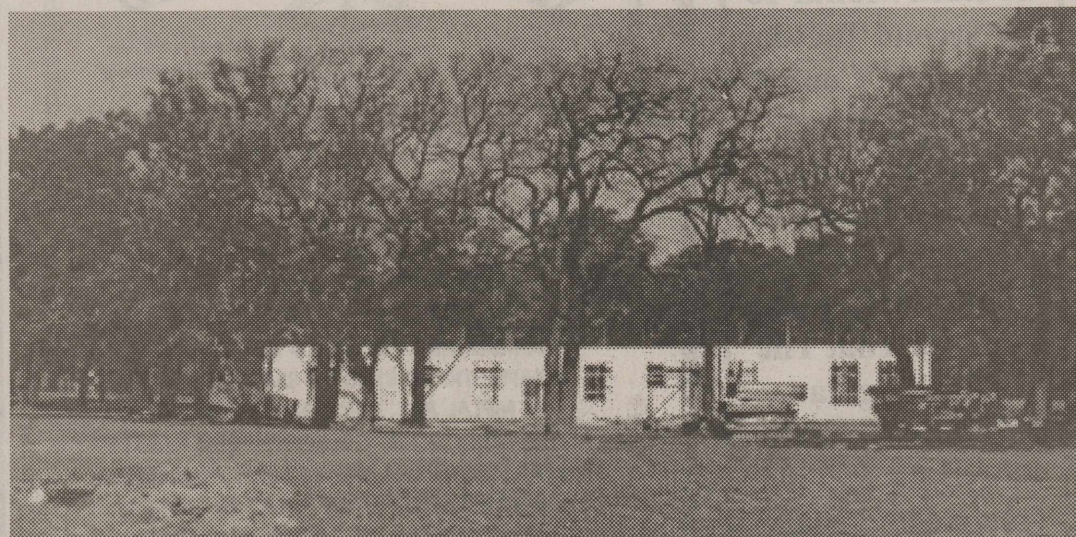
BACKSIDE OF CHARLES AND KATHY CHESHIR HOUSE The walls have been constructed.
