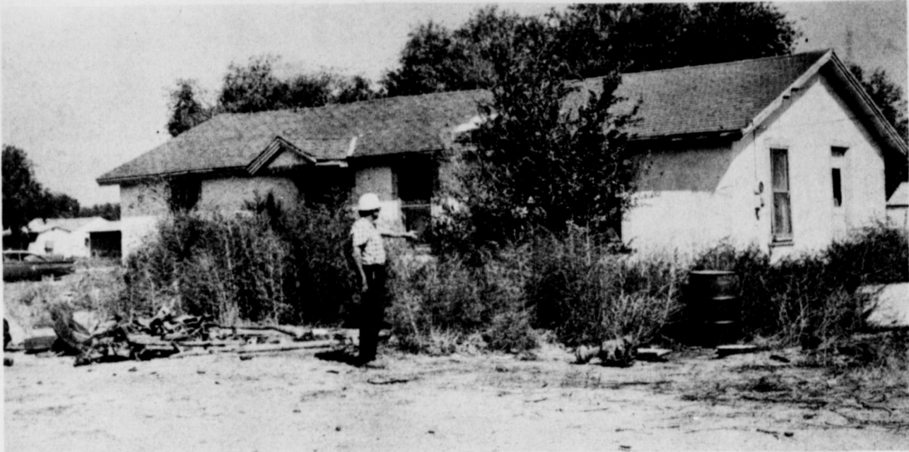
EMPTY HOUSE--"This vacant house, with trash and weeds, could cause a fire," warned Marshal Jones. "A rash of fires," said Jones, "could result in loss of life, or property and cause an increase in Muleshoe fire insurance rates. The city should take the steps to correct this by ordinance," Jones said.
