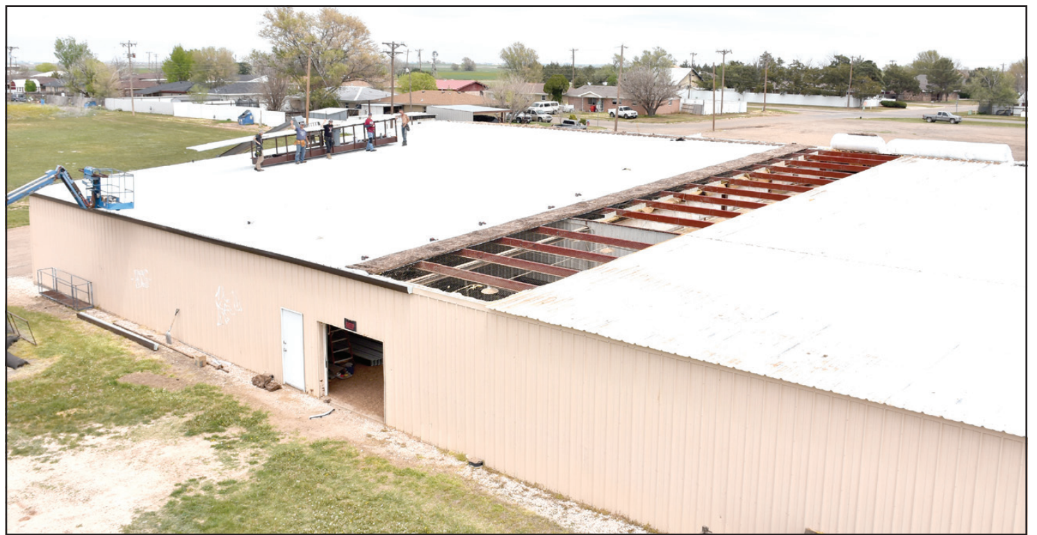
The Friona Community Center is finally getting a new roof. The 15,000 square foot structure was built by Lewellen Construction of Friona and hosted its inaugural event, the 26th Annual Parmer County Livestock Show, in February of 1974.
