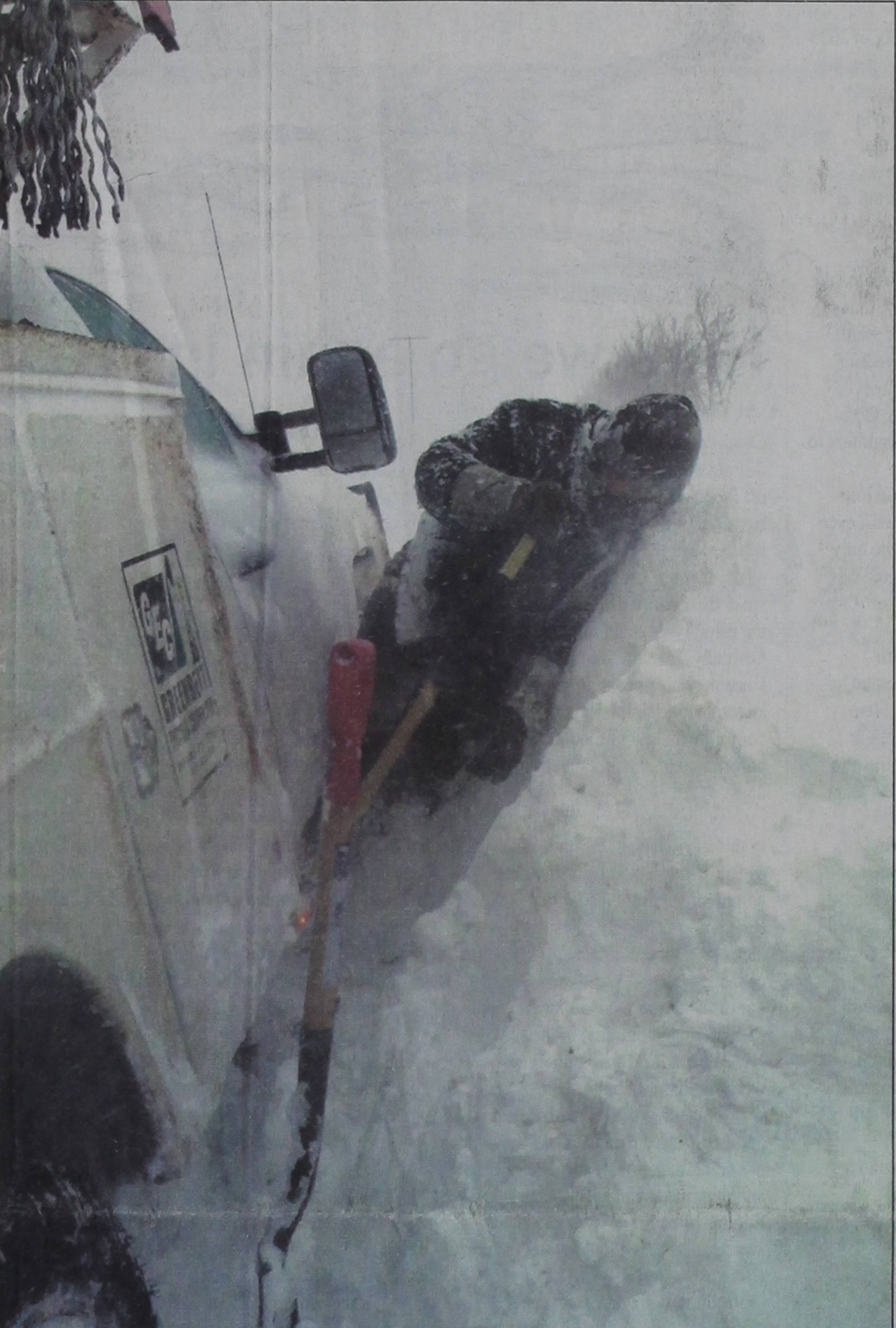
Greenbelt Electric Cooperative employee Levi Proaps works to dig out a service truck while making line repairs in Wheeler County Monday.
