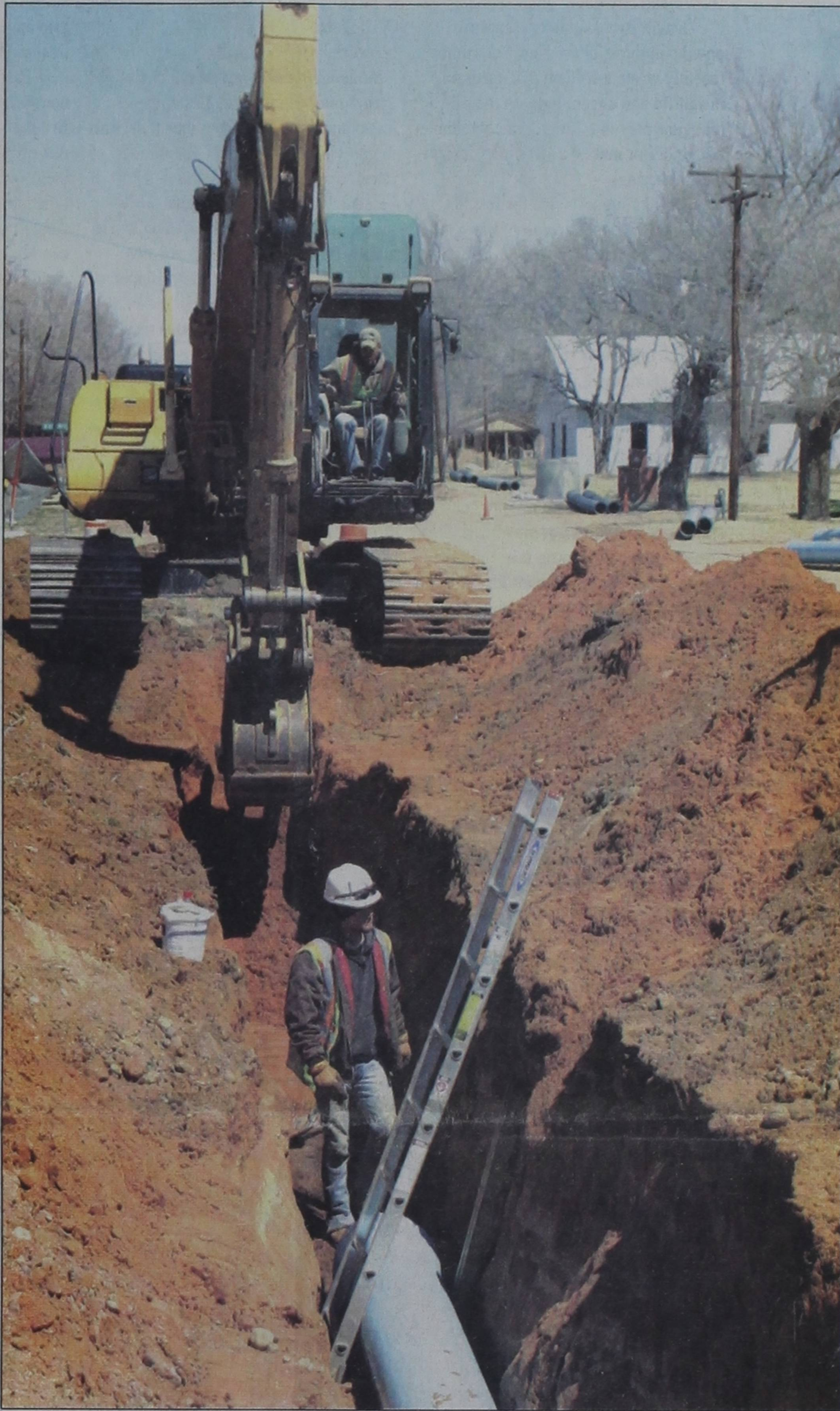
Workers install pipe for the Greenbelt groundwater project Monday on Sully Street in Clarendon.
