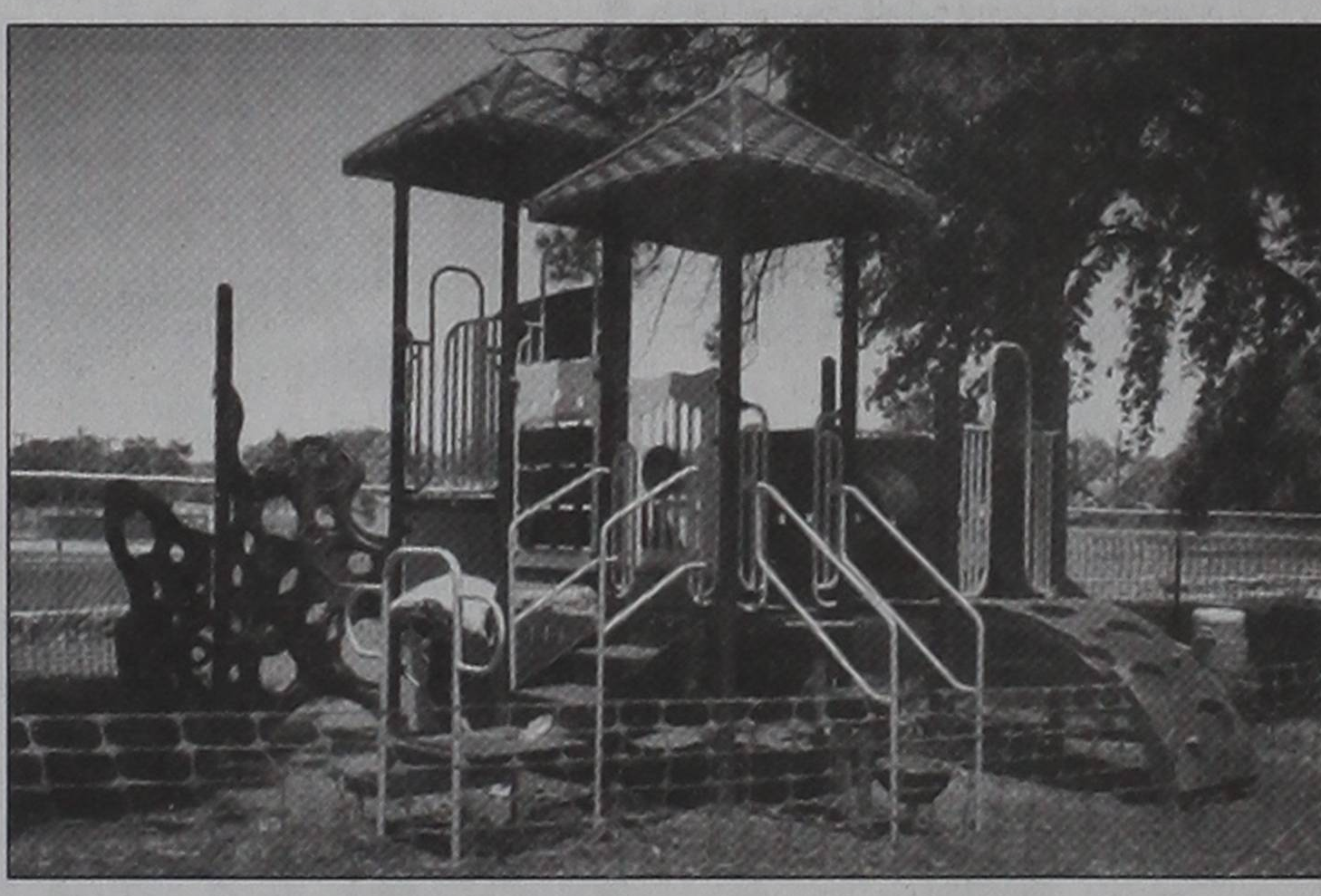
Chance Mark Jones memorial playground is currently under construction in Prospect Park and is set to be completed before July Fourth.
