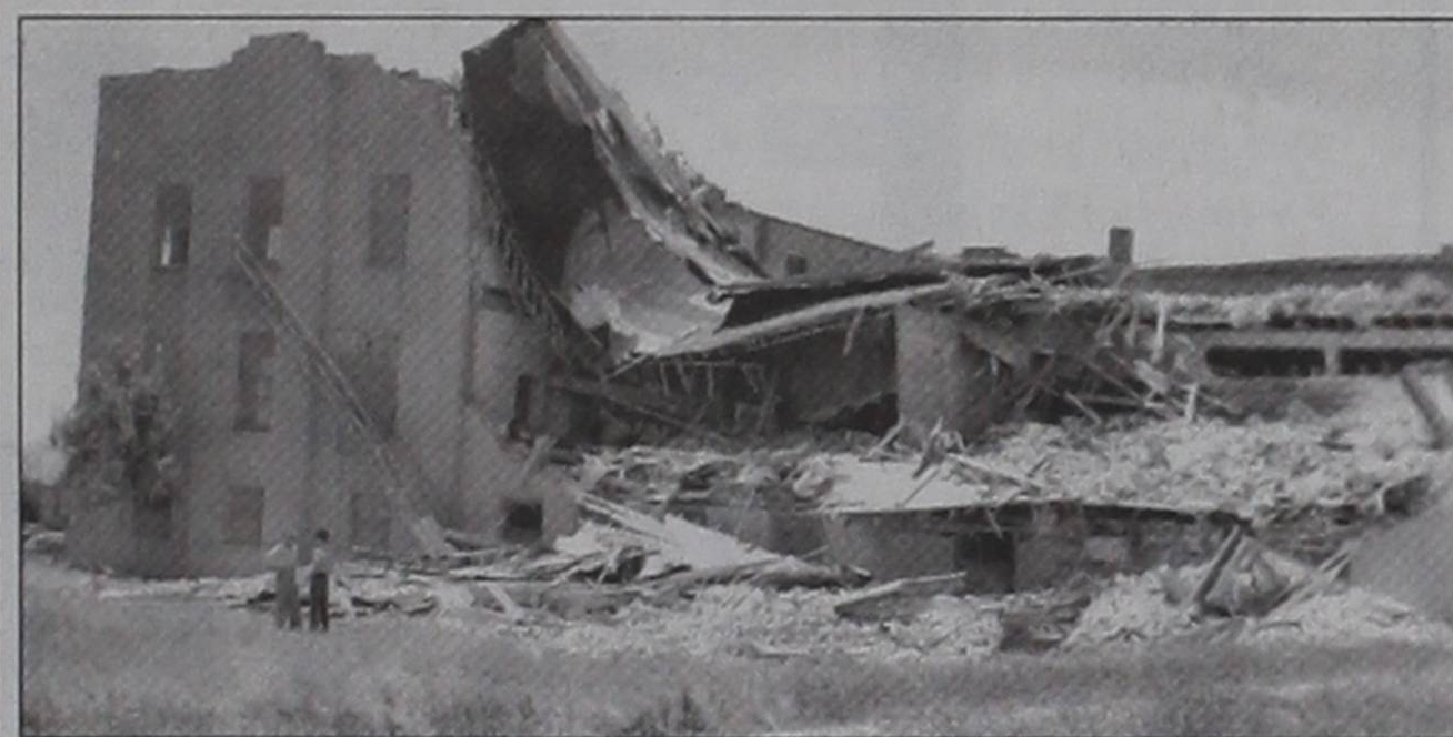
Looking at the north side of the Girls Dormitory (the current Old Gym), a bomb blast could hardly have done worse damage to the building's north wing. Other sections of the building did not collapse but were torn and wrecked.
