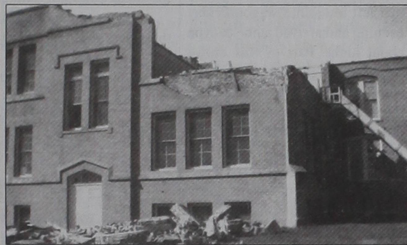
The rear of the College main building took most of the force of the tornadic wind. Walls and partitions throughout the building were cracked and distorted, and much valuable equipment was damaged by wind and water.
