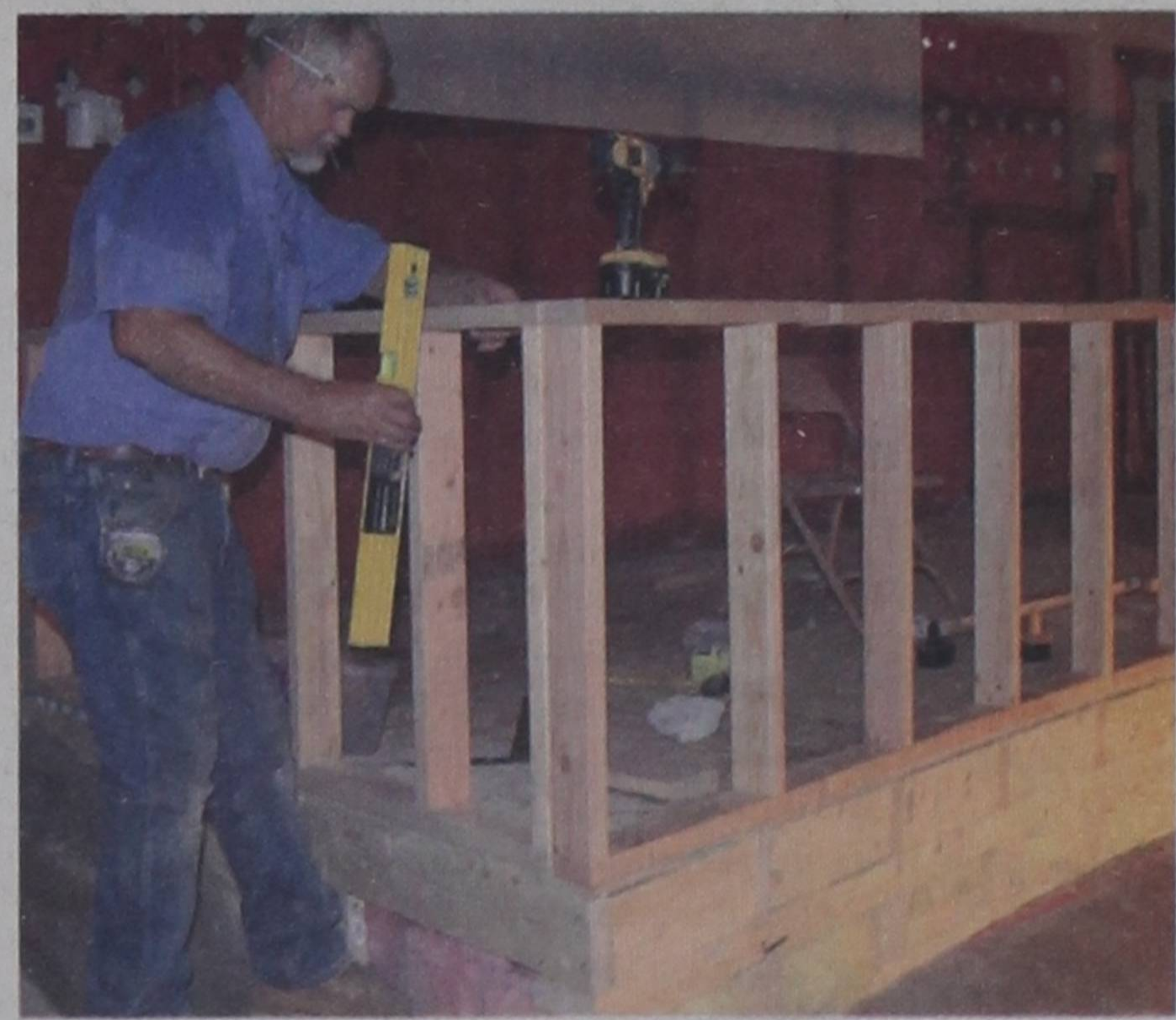
Leo Brewer works on the new handicapped seating area at the Mulkey Theatre Tuesday afternoon.
