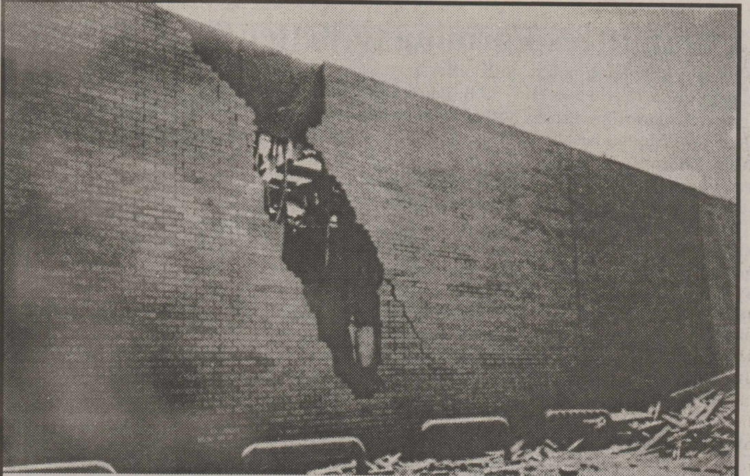
TORNADO RIPS HOLE INTO SIDE OF VILLAGE MARKET — West wall of store suffered major damage. This section of the city received the most destruction during the storm.
