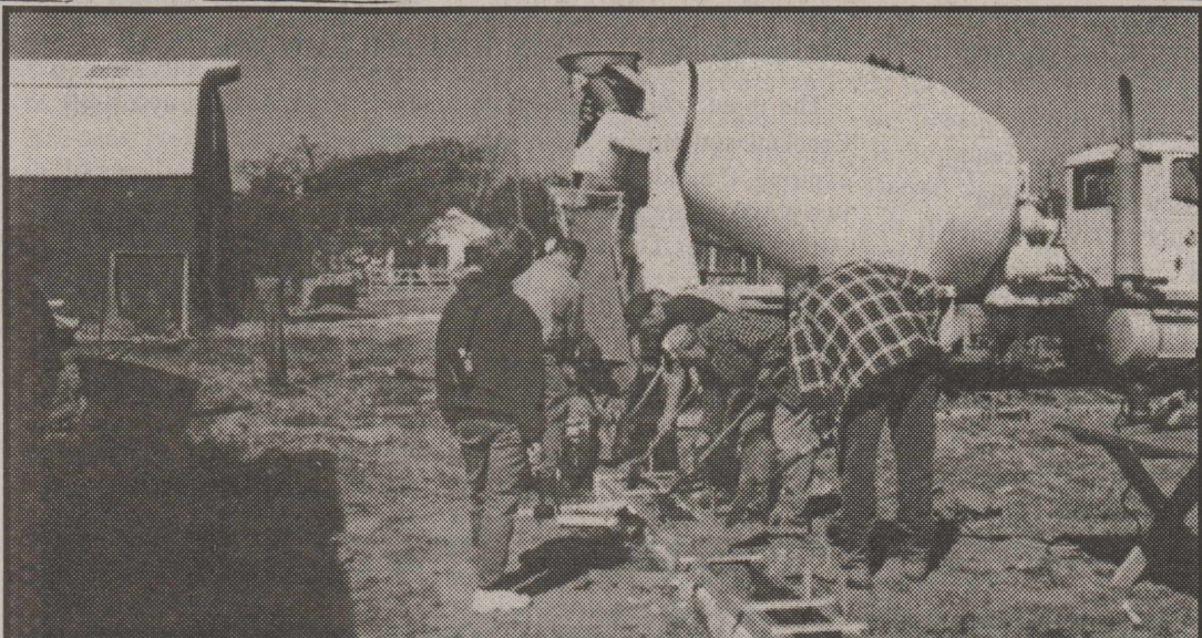
COTTONWOOD FIRE VOLUNTEERS POUR CEMENT FOR NEW FIREHOUSE— Various members of fire unit busy at pouring concrete and getting ready to erect metal building that will be the new Cottonwood Fire House. (Photo by Wallace Bennett.)
