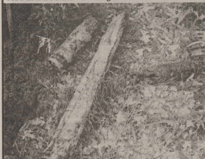
COLLAPSED SEWER LINE— Orange berg pipe, used in the 1940's.
