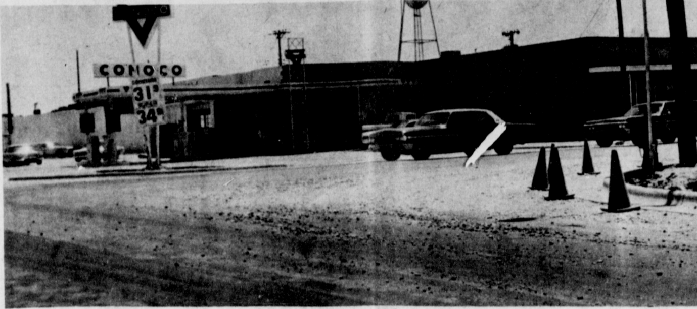
CROSSROADS INTERSECTION IMPROVEMENTS WELL UNDERWAY--Despite brief motorist inconvenience during the past week, the massive intersection improvement at the Crossroads at Highways 70-84-214 is progressing rapidly at this time. Pic-
