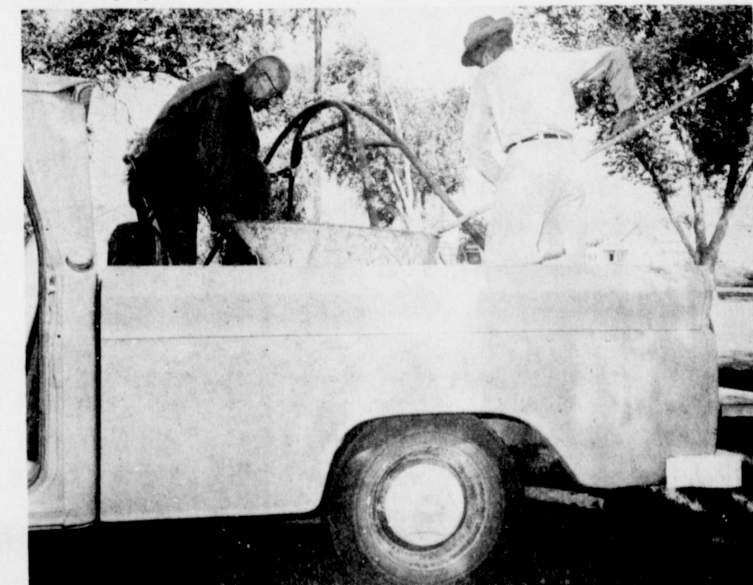
NEW PARK EQUIPMENT--Rev. Walter Bartholf, left, Muleshoe Park and Recreation chairman and George Haskins, right, Muleshoe City employee, work mixing concrete in the East Side City Park. They are busy setting up new park playground equipment which has been received.
