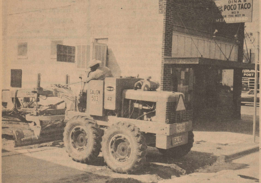
NEW BUSINESS TO OPEN IN DOWNTOWN OZONA - Dina's Poco Toco will open its doors at 10 o'clock tomorrow morning offering a variety of Mexican Food. The business is located in the Nettleton building at the highway intersection. Under construction above is a driveway to enable patrons to pick up orders at the drive-in window. The Poco Toco will be operated by Mr. and Mrs. Luis Martinez.
