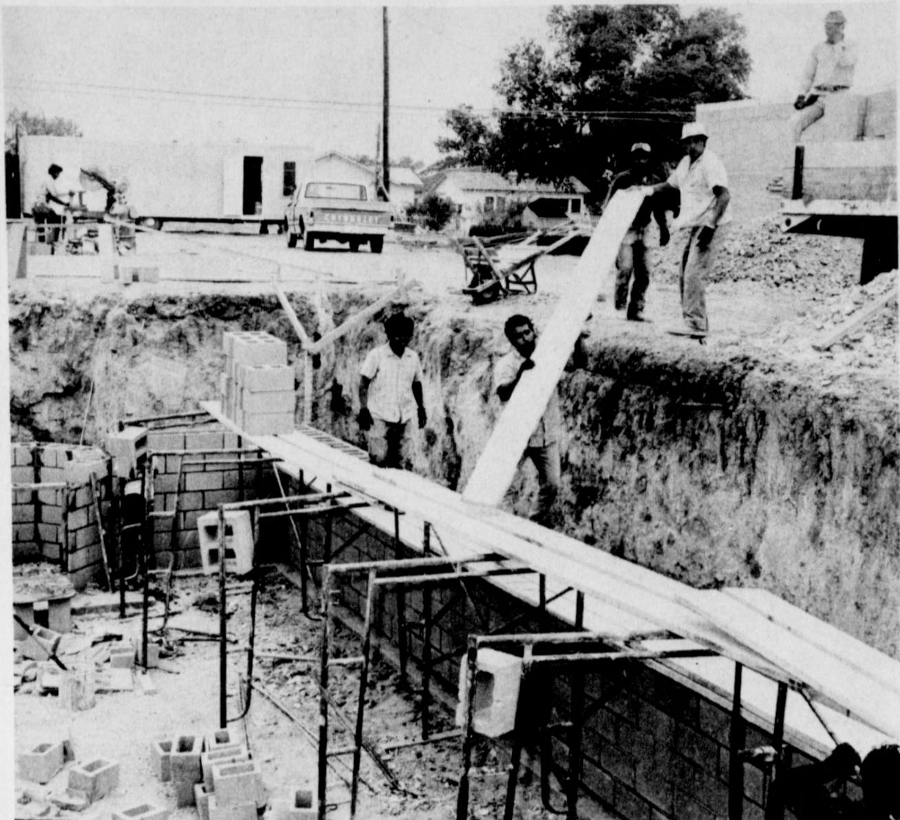
LIBRARY WALLS ARE GOING UP--Construction on basement walls at the new Muleshoe Area Public Library are well underway, with workmen from Lubbock shown as they prepare to unload another stack of concrete tile used in the construction. Jerry Galley, contractor from Lubbock, has his workmen busy
