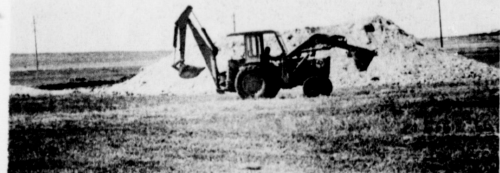
MYSTERIOUS HOLE AT NEW PARK SITE EXPLAINED . . . Several people driving down West Avenue D have noticed this huge hole and pile of dirt at the new Muleshoe City Park site and wondered what it was to become. City Manager Albert Field reported to the Journal that the city is digging the hole and using some of the cliche out of it for general road repairs in the city. Some of the cliche will also be used for paving roads on the park site and other construction work there. The city plans to develop the hole later into a small pond on the park site.
