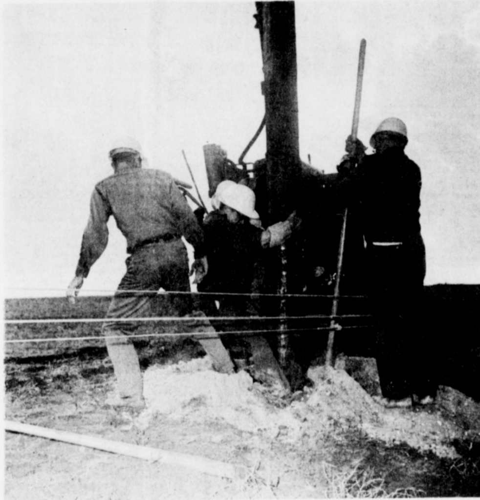
WORK CREW REPAIRS TORNADO DAMAGE . . . Work crews from Bailey County Electric were out Sunday repairing damages to electric lines between Circleback and Needmore following a tornado which dropped down in that area around 4:45 p.m. Sunday afternoon. Other damages from the tornado included a storage building and fences on the F.W. Wall farm southeast of Needmore.
