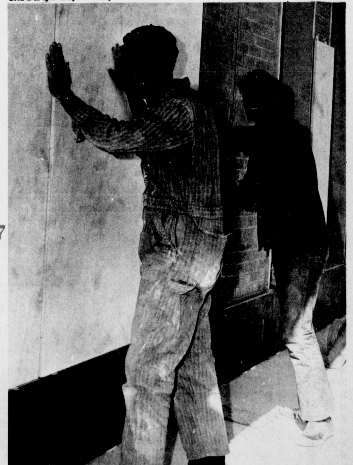
MARBLE BEING PUT UP . . . . Workers were busy this week placing the Alabama Marble at the New Tri-County Savings and Loan Association on Main Street. The new location for Tri-County should be completed by April.
