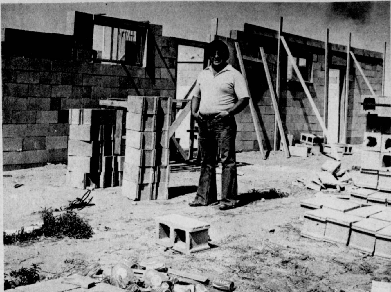
CONSTRUCTION UNDERWAY ON HOUSING...Ramiro Perez of Robert Ruiz Inc. is shown with a portion of the housing units being constructed just to the southwest of the Robert Ruiz Inc. vegetable
