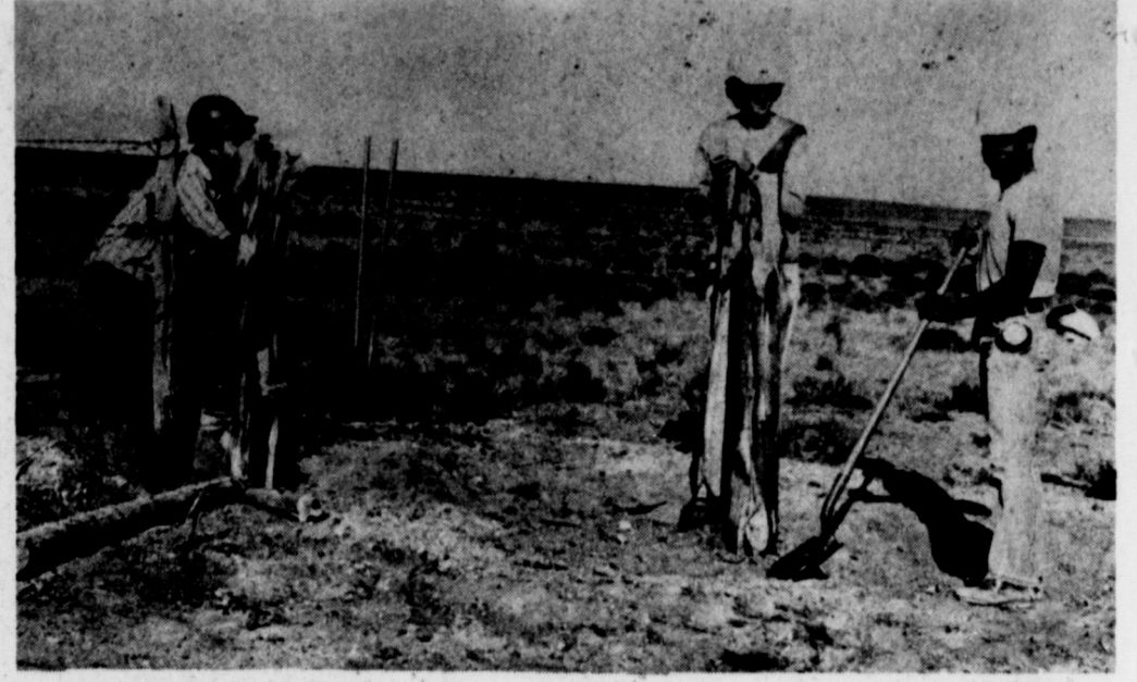
SETTING POSTS...As Mario Mendez, Texas A&M Student from Dallas sights, Billy Vinson, Muleshoe and Johnny Rosemond, Amherst, prepare to set another post for the new fence under construction at the Muleshoe National Wildlife Refuge. The students will do additional work during the next seven weeks.
