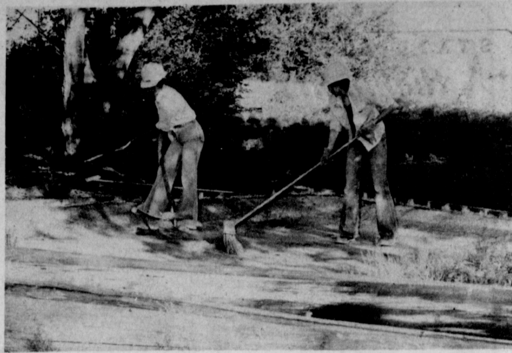
CLEANING IT UP... Susan Masten, Morton and Millie Roberts, Enochs are two of the twenty students and six summer staff members who are helping with the clean-up and repair work at the Muleshoe Wildlife Refuge this summer. They are cleaning out the fish pond, preparing for restocking.
