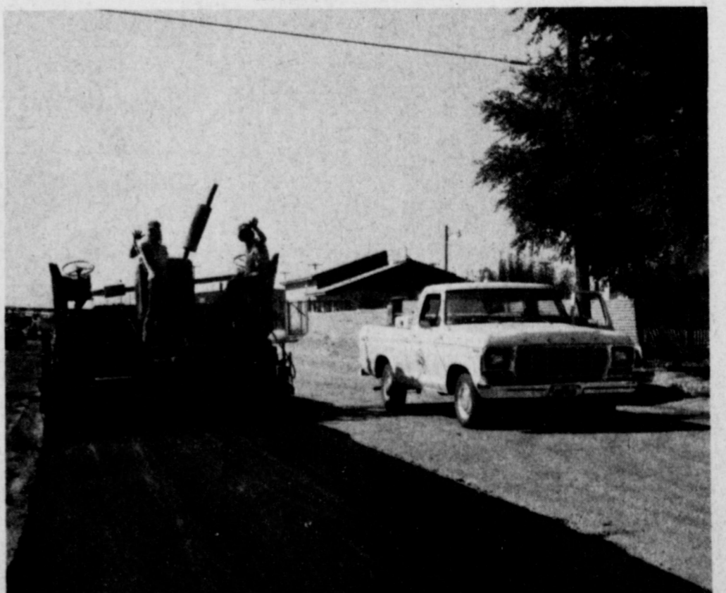
SEALCOATING AND REPAIRS --Workmen from Jake Diel Dirt Moving and Paving have started some sealcoating and repairing of streets in Muleshoe during the past several days. The operation follows complaints from residents who said paving operations were insufficient in several areas of the city. A final payment to Jake Diel was not authorized until all the work was completed satisfactorily.
