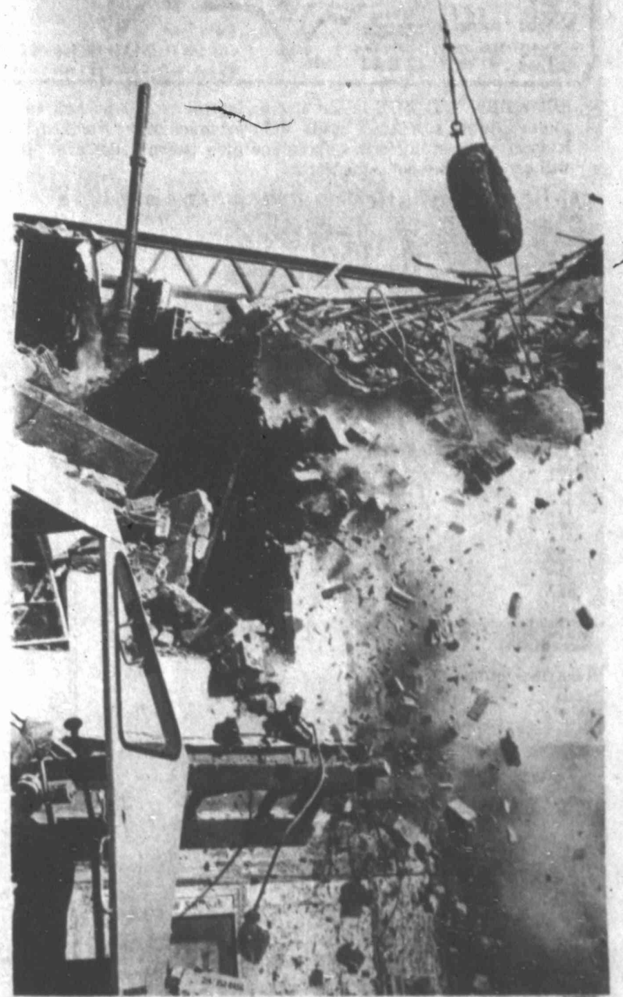
THE TWO-TON wrecking ball makes a demolition-derby fare out of the old Tower Theatre off Main Street in downtown Midland. The building will be replaced by a parking lot.
