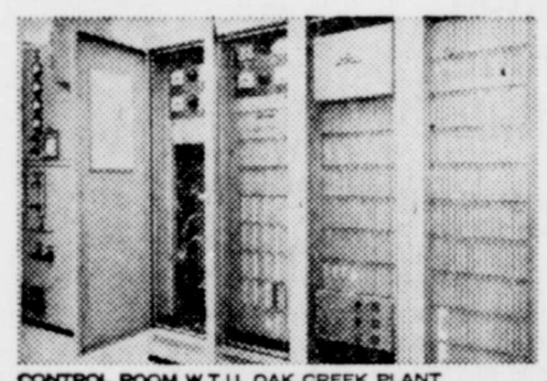
CONTROL ROOM W.T.U. OAK CREEK PLANT
