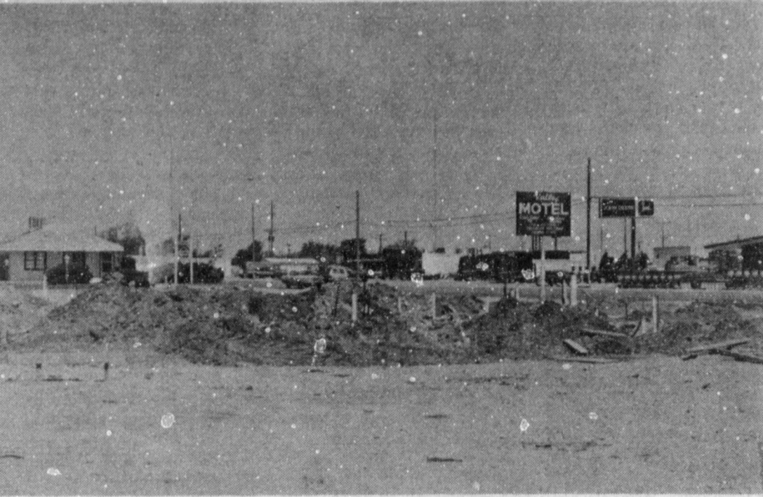
NEW EATERY IN TOWN -A fish and chicken fast food service is currently being built on American Boulevard in the previous location of Puckett and Clark Trucking. Groundwork is now being laid and construction should be completed in the not too distant future.
