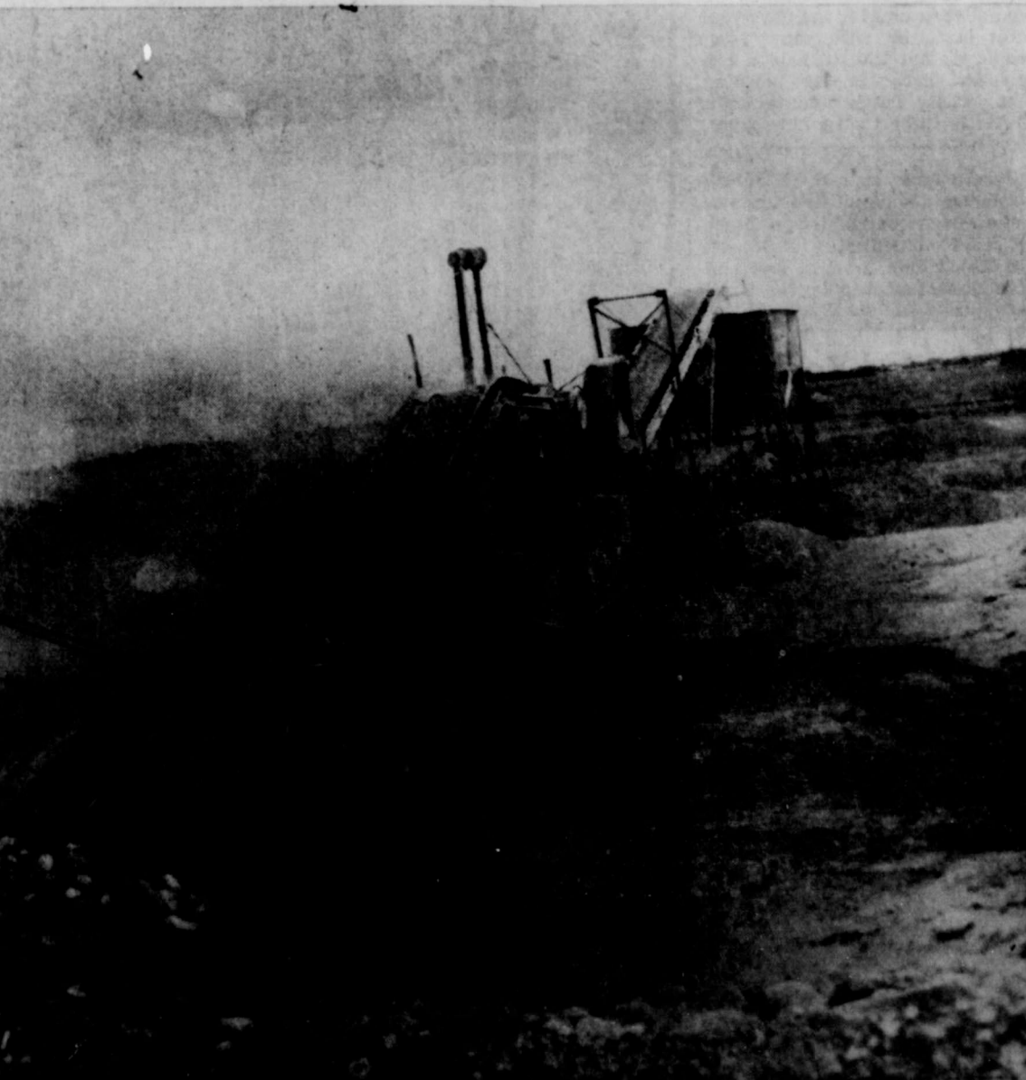
FAST PROGRESS on Artesia's First Street highway project has been made possible by the mighty maw of this stone crusher. Roaring away at the Longenbaugh & Coe installation beyond the airport, the huge crusher provides road material at an amazing pace. Despite delaying rains, the construction has kept ahead of schedule. (Advocate Photo)
