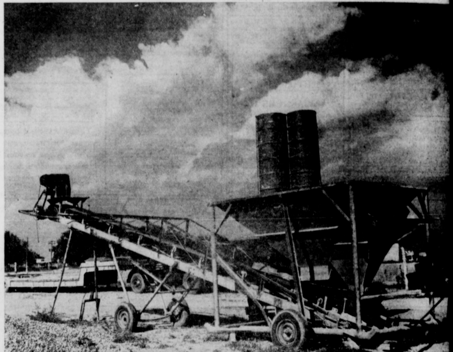
GLAMORIZED BY CLOUDS stands the huge concrete mixer that prepares the concrete used by the company. Local ingredients are used as far as possible, gravel from nearby pits and sand from near Roswell. The concrete must meet strict specifications set down by Stiver. From the mixer, concrete goes into the mix trucks that take it to the job. The Concrete Ditch Liners Co. have been in business here three years but moved to the Hope highway location only recently. (Advocate Photo)
