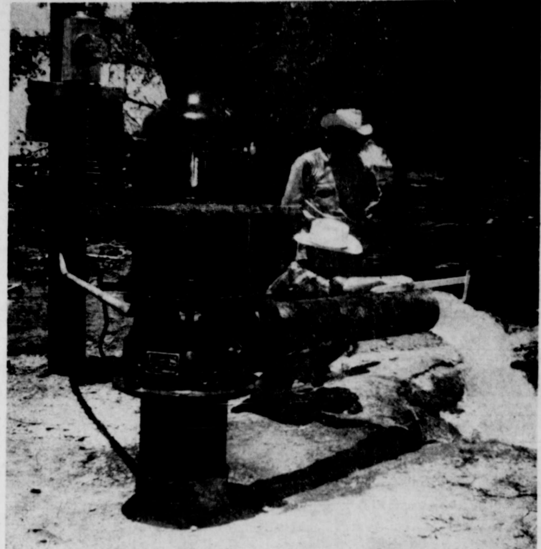
BIG PUMP —This 1,500 gallon per minute irrigation pump is used on the Joe Lee farm, south of Artesia. It was installed by the Bristow Pump Co. of Artesia and is a U. S. Electric Motors, Inc., product. Standing is Mr. Lee, while kneeling to measure the water flow is Sam Coates, a Bristow Pump Co. partner.
