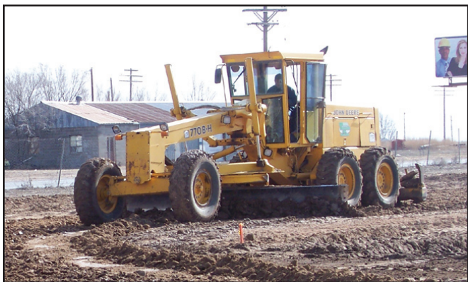
Work begins on Bailey County Electric Co-operative's new offices located on E. American Blvd.
