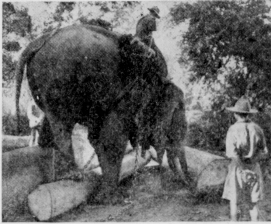
Sometimes the highly mechanized service of supply of the U. S. army finds it can do it better with animals. In Burma, for instance, Indian elephants, directed by native mahouts, handle large logs used in military construction. Here a big tusker pushes a log down the sloping bank to the river. The timbers are lashed together to form large rafts, which are floated down the Irrawaddy to Myitkyna. (Signal Corps Photo)
