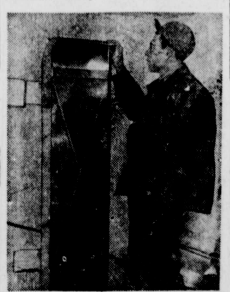
Arthur Miller of Union, Ill., admires the new heater recently installed in his milk house.
