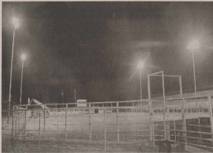
CALLAHAN COUNTY SHERIFF'S POSSE RODEO ARENA MAJOR LIGHTING AND ELECTRICAL PROJECT NEARING COMPLETION.
