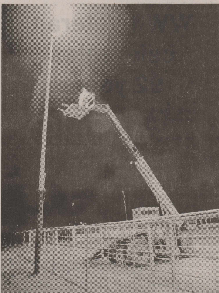
CALLAHAN COUNTY SHERIFF'S POSSE NEW LIGHT POLES BEING ADJUSTED FOR MAXIMUM ARENA LIGHTING.
