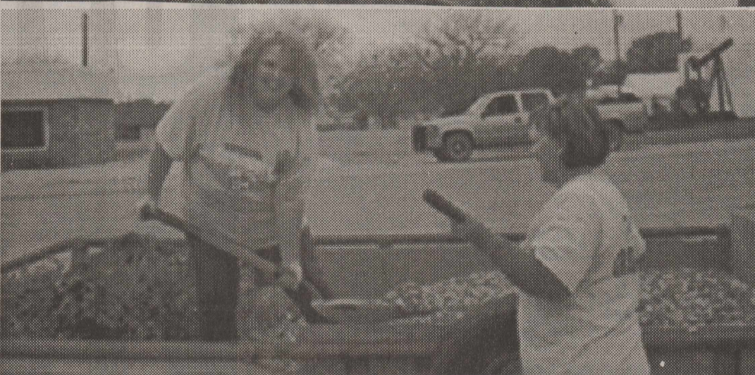
Pictured left to right, Lajeana Hayes- Long and Delynn Purviss shovel gravel.
