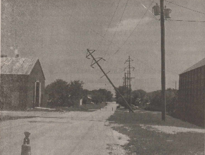
Damage to telephone and electric poles.
