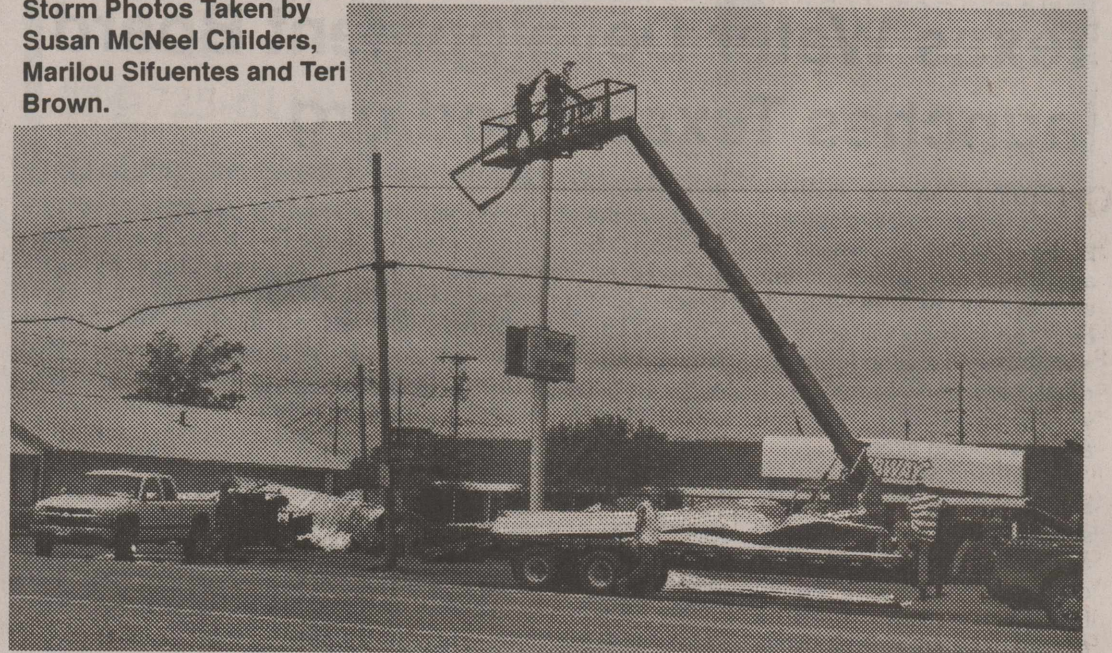
Removing the frame of the sign and cleaning up the debris. By Friday afternoon the debris had been hauled away.
