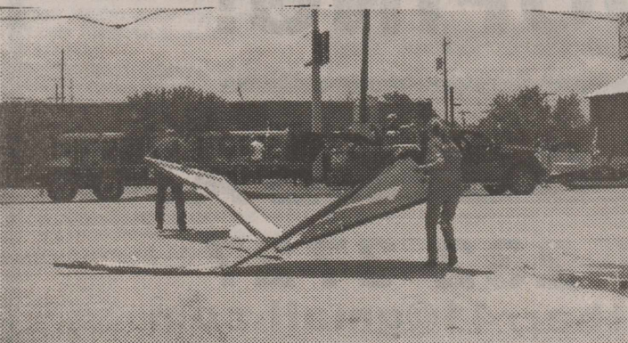
Removing pieces of the Subway sign from the Food Plaza parking lot.
