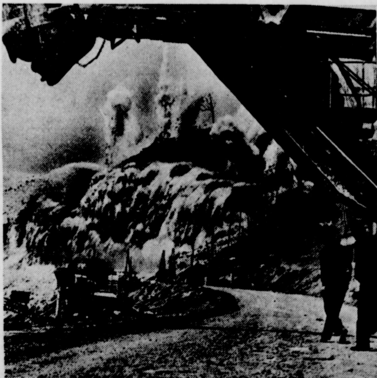
Here is one of the biggest booms ever! Sixty-two tons of explosives tear down a mountainside at the TVA Cherokee dam site, moving 450,000 tons of rock! The picture, framed by a huge shovel, shows nearly half a million tons of rock cascading down the mountainside, looking for all the world like a huge waterfall.
