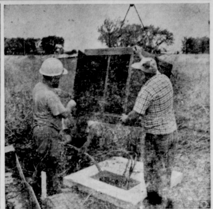
Weighing only 666 pounds and 28 1/2 inches high, an Allis-Chalmers transformer installed in a Janesville, Wis. subdivision is easily maneuvered into place on its concrete pad. The subdivision is the first in the state with both electrical and telephone wires buried together in a common trench. The underground wiring system eliminates overhead poles and wires. Allis-Chalmers acted as general contractor for the entire project.
