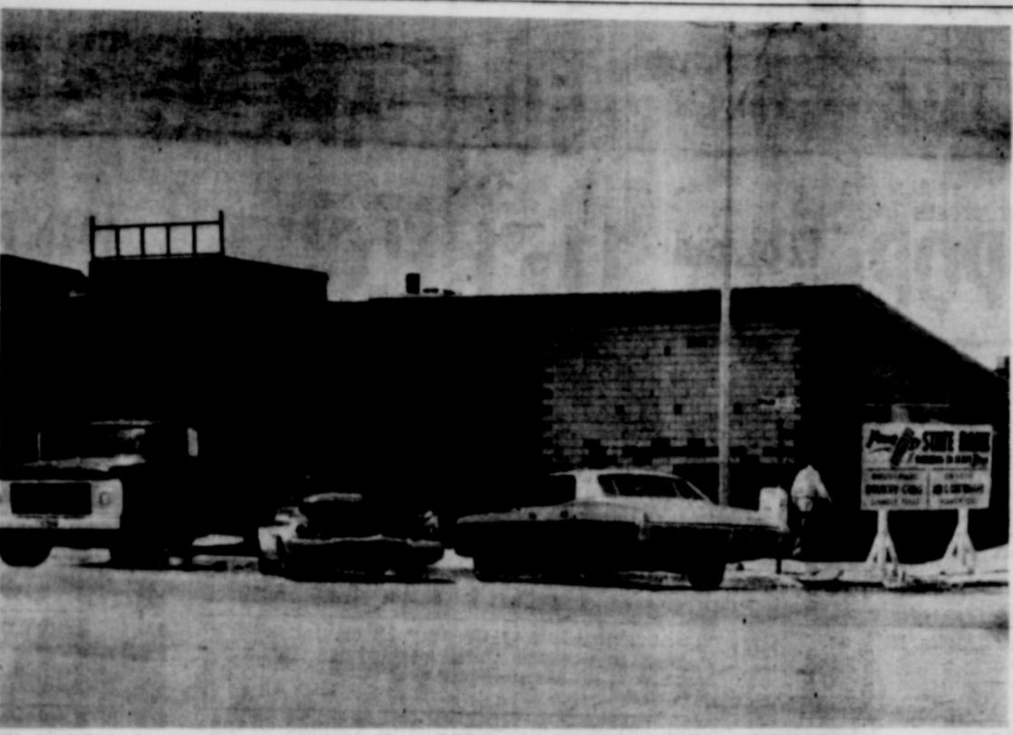
Remodeling is progressing on schedule at the First State Bank in Silverton, with construction continuing on the exterior while workers begin finishing the inside of the new portion which will include a meeting room for community.
