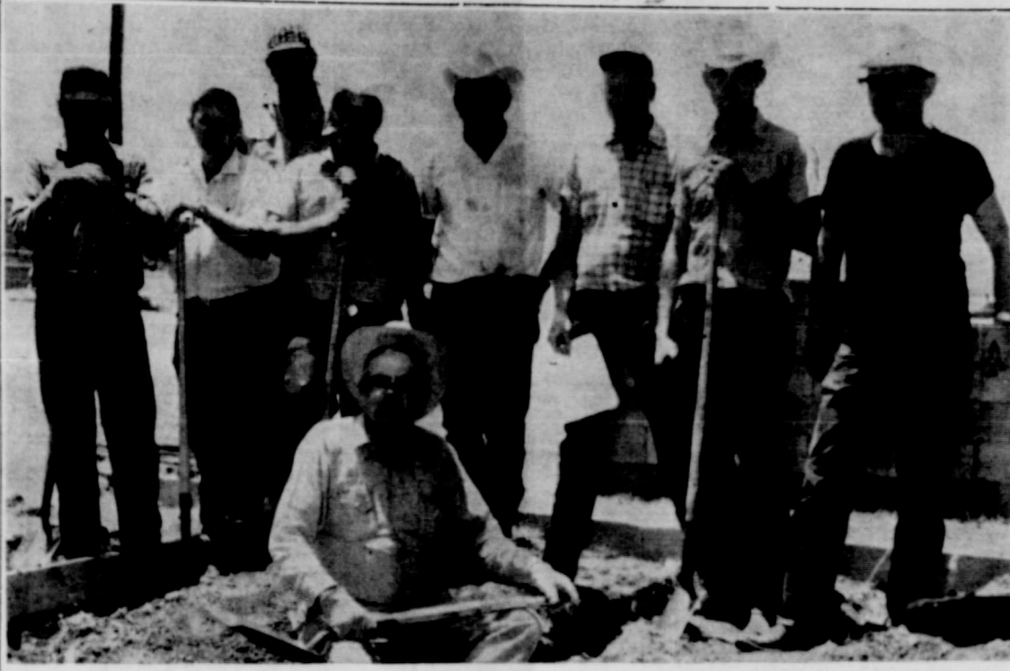
Construction is now underway on restrooms at the football field, a project undertaken by the Silvertown Young Farmers with public support. The chapter members shown assisting Charlie Holt, seated, are (from left) Alton Riddell, Robert H. Hill, Charlie Parker, Calvin Shelton, Guinn Fitzgerald, G. W. Chap-pell, Jimmy Myers and Dwain Henderson.
