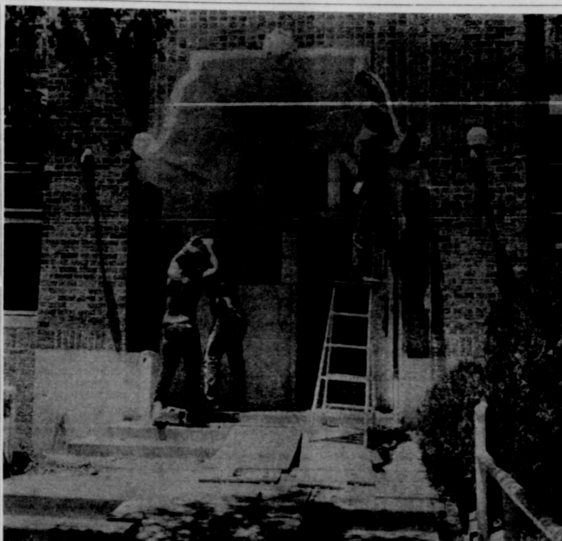
Workmen were pictured last week as they exterior while a total remodeling is more than half completed inside. Workmen foresee New Aluminum-frame windows have added no problems and expect to be finished with a fresh new appearance to the building's the remodeling before school starts.
