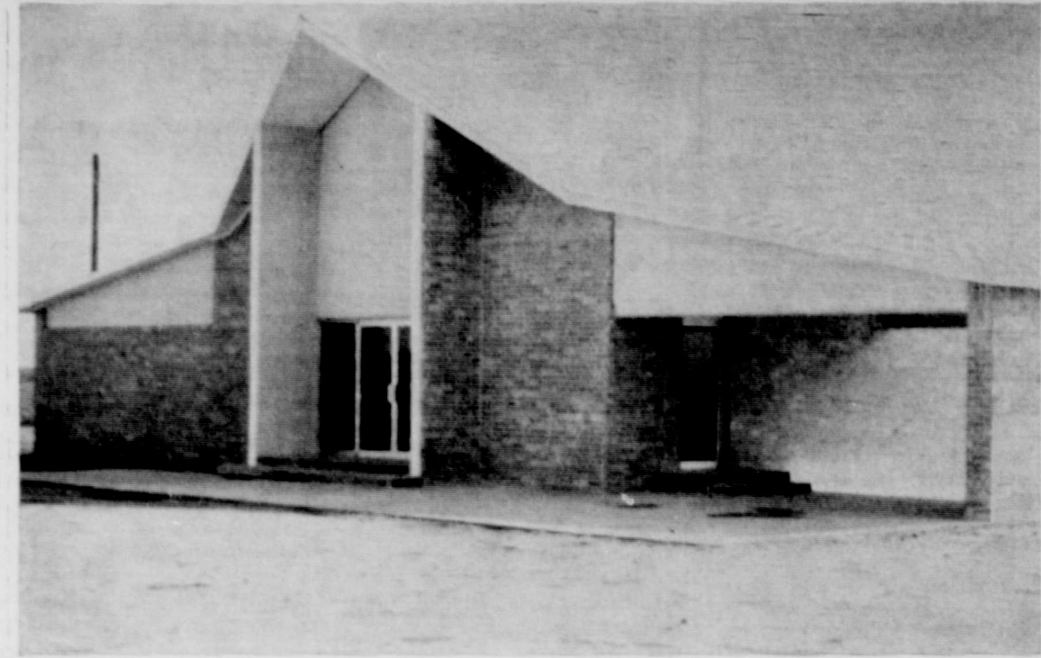
Work is still going on in the remodeling of the Rock Creek Church of Christ. A fellowship hall has been added, part of which will be divided from the auditorium by an accordion partition which can be opened to seat a larger congregation for special occasions. A covered driveway has been added on the south side for discharging passengers from car to the church in bad weather. Work on the church was planned and carried out by the men of the church under the direction of the minister, Earl Cantwell.
