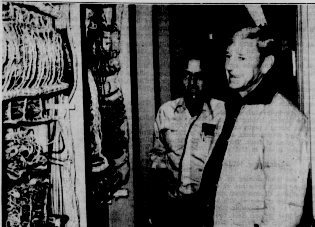
Billy Ray Ford and Jimmy Stone of General Telephone Company of the Southwest are shown with the new and expanded office equipment, the latest electronic switching equipment available to the industry, which was delivered to Silverton last week.
