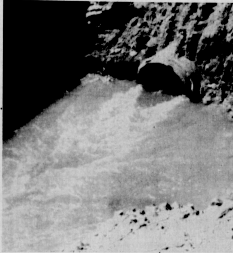
Shown is the 30-inch pipe which has been letting the floodwaters past Mackenzie Dam so that construction work on the dam can continue.
