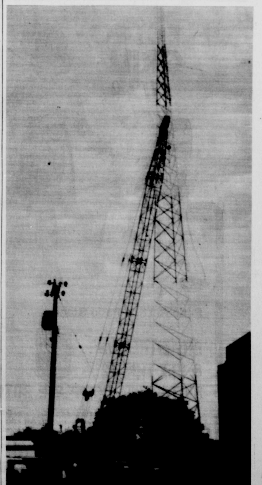
Briscoe County's new communications tower was raised Monday morning by a large crane which made quick work of the task. The modern communications system will be for use by the county sheriff's department and the City of Silverton. The project will link 25 county and 45 city law enforcement agencies and will cost a total of $1,188,185.00, seventy-five percent of which is to be paid by the Texas Criminal Justice Council.
