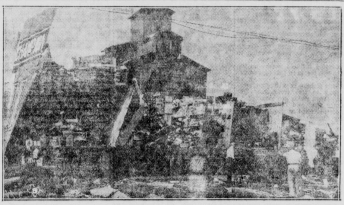
This is a wholesale grocery firm in Brownsville, Texas, of what is left of it after sad collision with a tropical hurricane, the worst ever to visit Texas' garden spot, the Lower Rio Grande valley. The twisting wind tore the building to pieces, the driving rain ruined and waterlogged everything. Scenes like this are not the exception but the rule, as one surveys the storm area.
