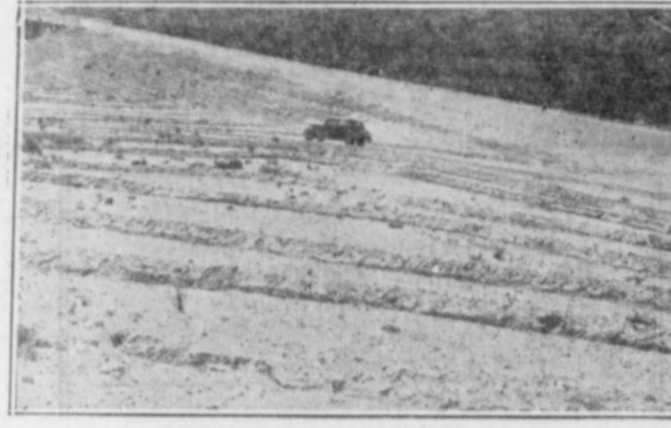
Work enacted in French's article includes level terraces on slopes of highway fills and cuts to prevent soil erosion as in the picture above on Highway 1 five miles west of Big Spring.
