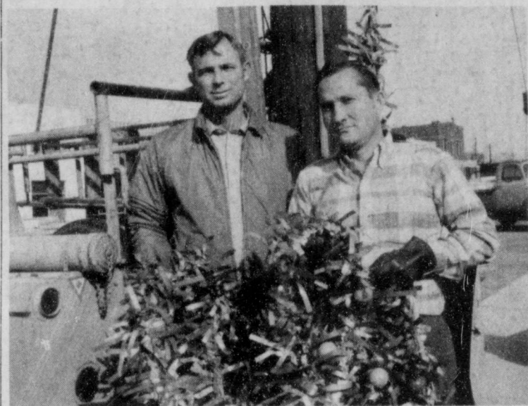
Stringing Christmas lights in Rotan Wednesday were Garvis Hinso and Perry Thomson, West Texas Utilities Servicemen.
